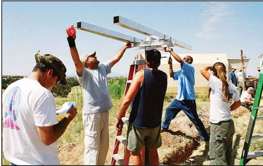
Students enrolled in SFCC's course "Summer Solar Intensive" help install photovoltaic solar panels at the college's ECDC in July 2007. The panels generate electricity that the college sells to PNM.
