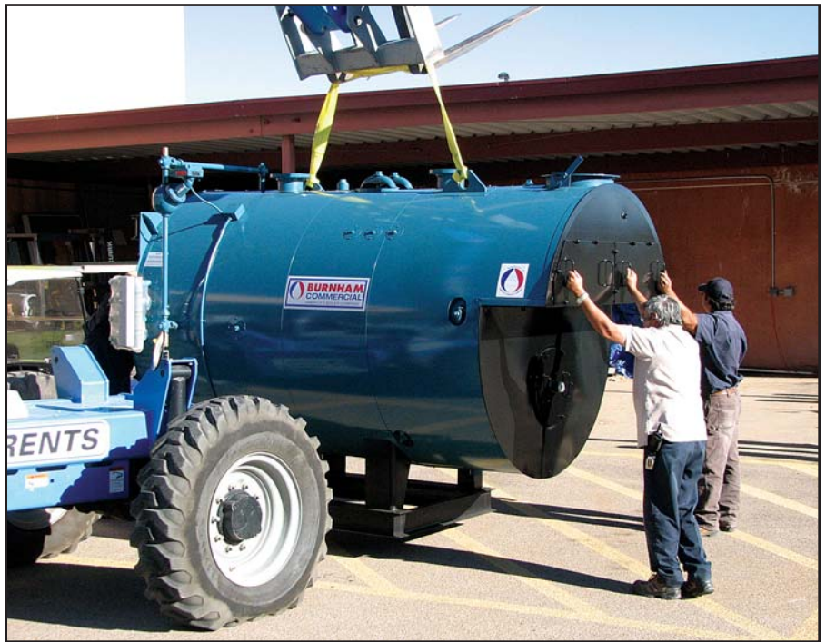
The college's plant operations receives delivery of the biomass-heating unit at the college's loading dock. The new heating system will decrease the college's dependence on its gas boilers.
